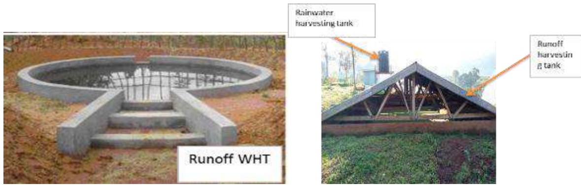
Figure 8-10: Run off water harvesting tank
