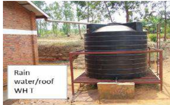
Figure 8-9: Rain water harvesting tank
