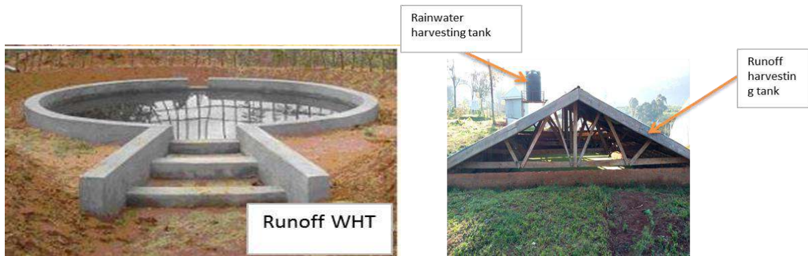
Figure 8-8: Run off water harvesting tank
