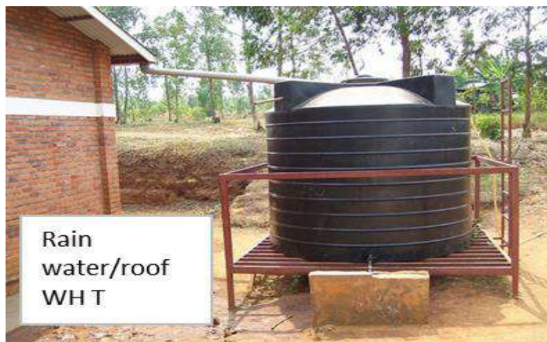
Figure 8-7: Rain water harvesting tank
