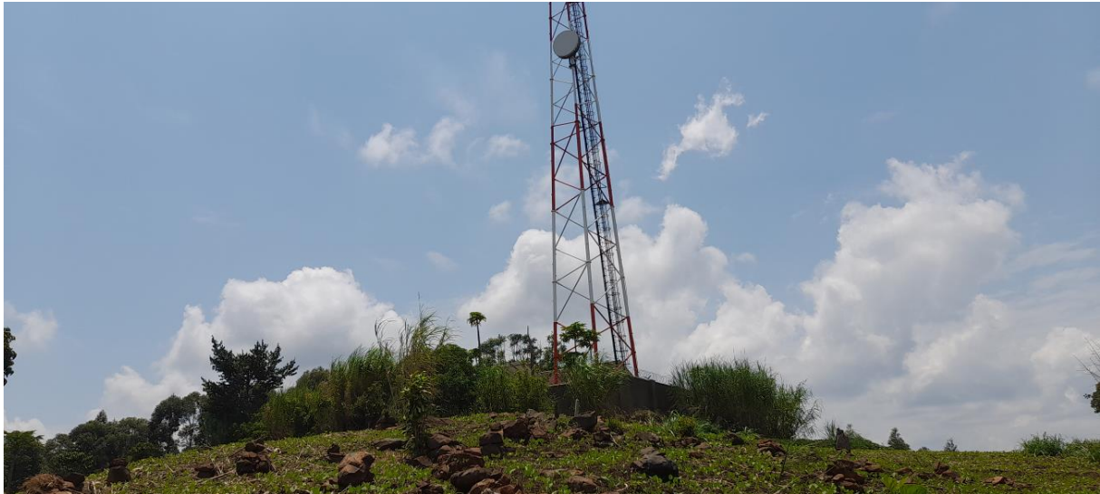
Plate 19: One of the Telecommunication masts within the project area for the network services
