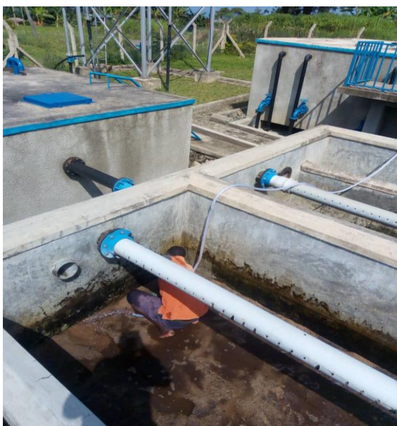
Cleaning of filtration chambers in Nyahuka to ensure supply of safe & clean water to
