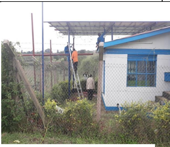
Installation of solar system on one of pump stations in Biguli-Kirinda town, Kamwenge district
