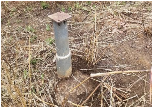
Drilled Borehole DWD 60632 – Wang Kenya 02 in Orom Sub county, Kitgum District
