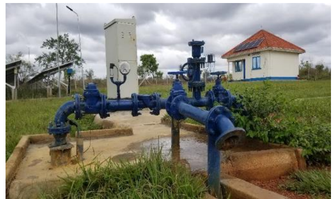
A developed Lugede Pumping Station (DWD 60596) in Acholibur, Pader District
