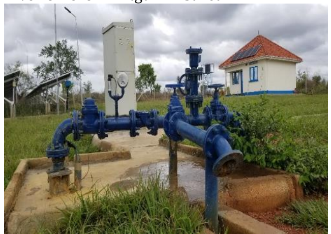
Existing pumping station DWD 60596 in Lugede, Acholibur, Pader District
