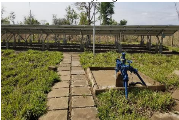
A developed Kakoo Pumping Station (DWD 61463) in Namokora Town Council, Kitgum District
