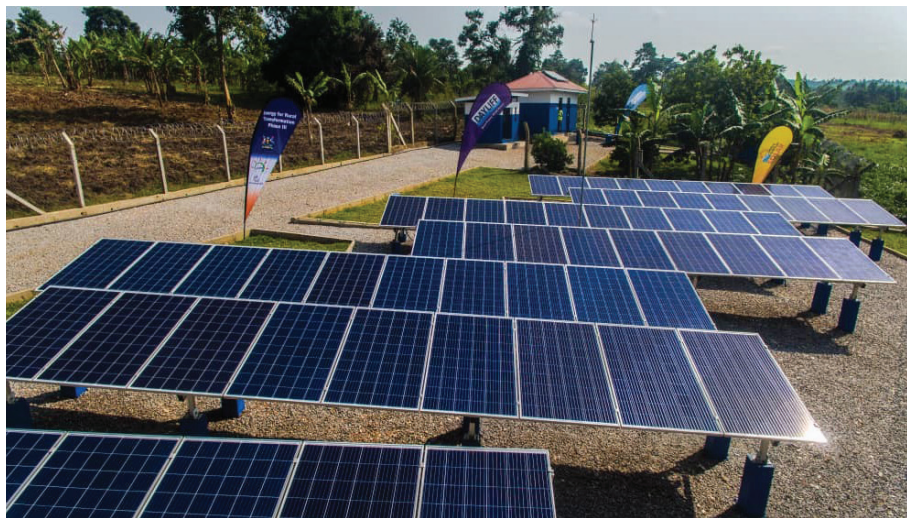
Well-Lined Solar panels to pump water for the community
