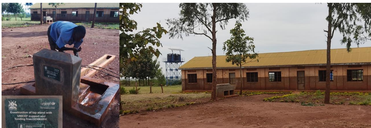
Figure 5-65: Piped water supply system (by GoU & UNICEF) at Tecwa primary school
