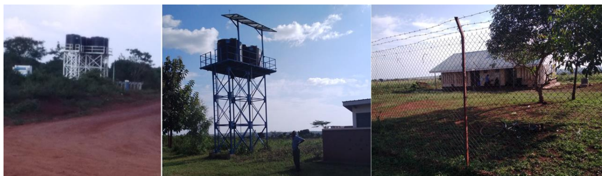
Figure 5-64: Solar piped water system that partly supplies Tecwa HC II (Latitude 1.52528024; Longitude 32.1183292)
